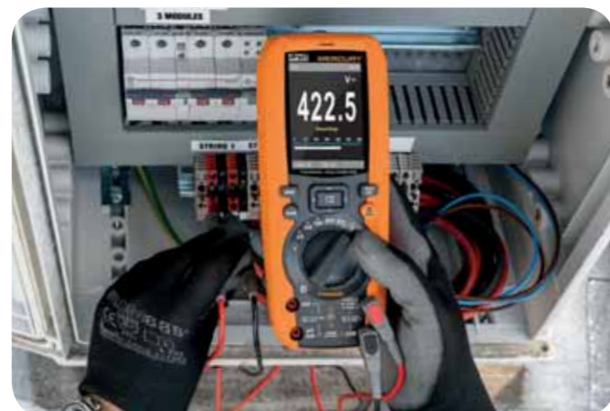
PV string Vmp measurement
