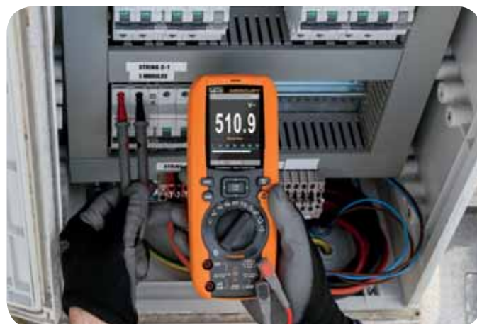
PV string Voc measurement
